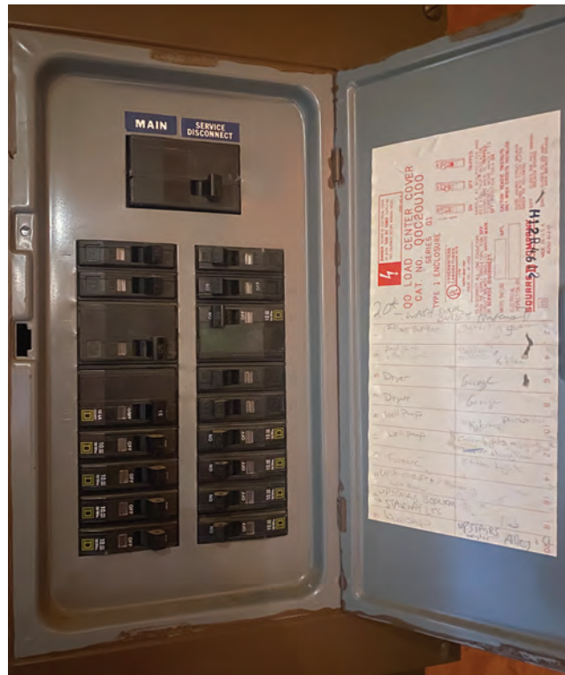
House circuit breaker (Image credit: Stephanie Lieblappen)
